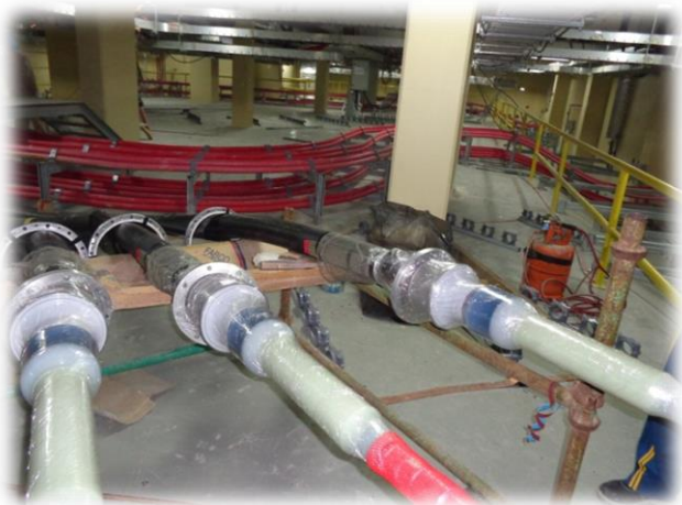
115kV EHV Cable Terminations Pfisterer ESG145
