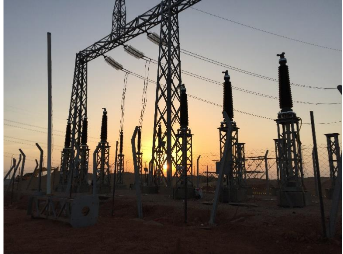
HV Cable Termination & Jointing
