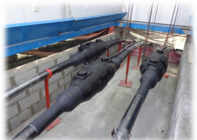
115kV EHV Cable Jointing Pfisterer Joints MSA145
