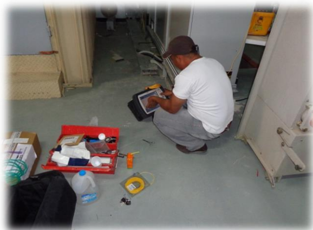
FOC Final Test Single Mode Ss 8907 In South Hail to Ss 8173 in Riyadh CN: 11031140/00 Contractor: CEPCO
