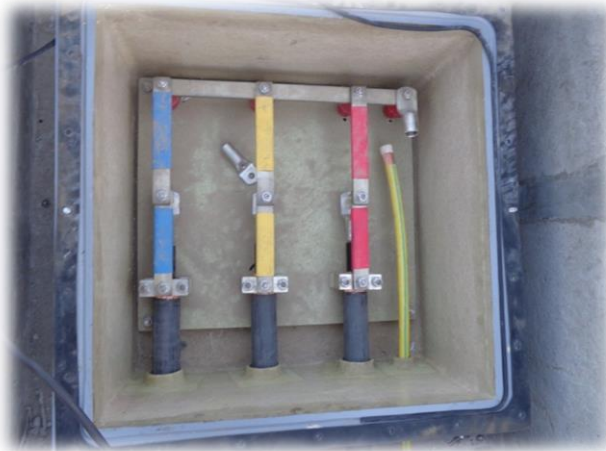
115kV EHV Link Box Terminations Al-Shaharani DC6P Direct Earthing Link Box
