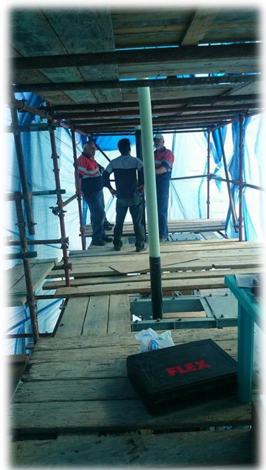
115kV EHV Outdoor Terminations ESP145 Pfisterer Make Contractor: Hadi Haider
