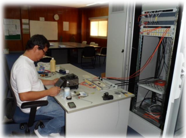
FOC Termination Tabuk Cement Contractor: Thyssen Krupp / Uhde Arabia
