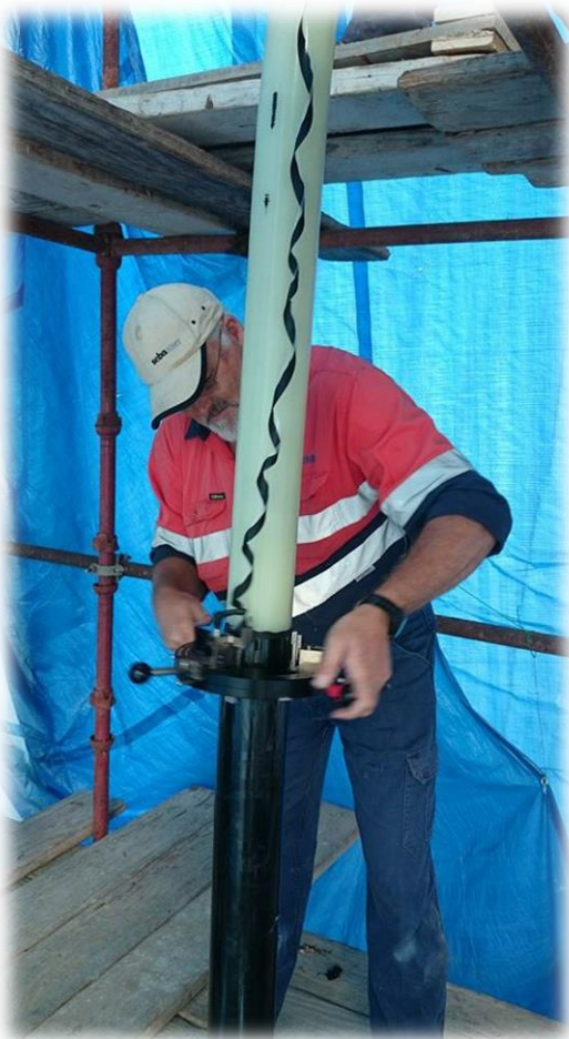
115kV EHV Outdoor Terminations ESP145 Pfisterer Make Contractor: Hadi Haider
