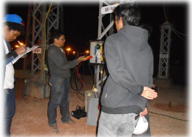
132kV Electrical / LV Testing Contractor: Al Babtain Contracting
