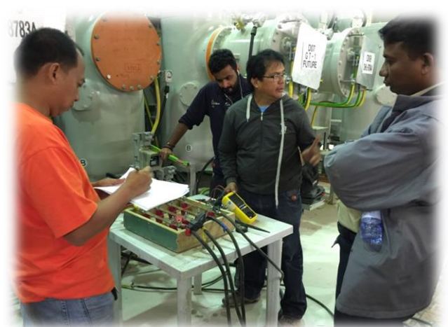
Positive & Zero Seq. Impedance Testing Contractor: Al Babtain Contracting
