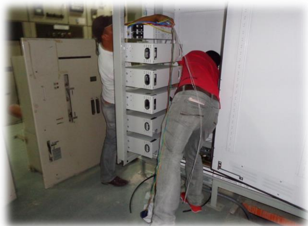
FOC Termination Single Mode Ss 8907 In South Hail to Ss 8173 in Riyadh CN: 11031140/00 Contractor: CEPCO
